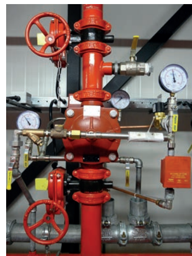
Fire system valves.
